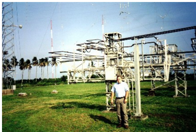
Transmitting Station Manager, Mr Charles Lewis, at the ground works of a 4x4 Curtain Dipole Array.
